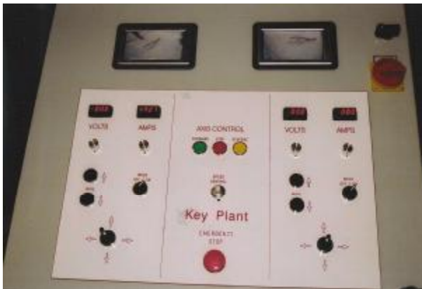
Central control station with 2 mini TFT screens
