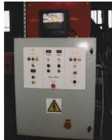
Central control station with 10" standard monitor
